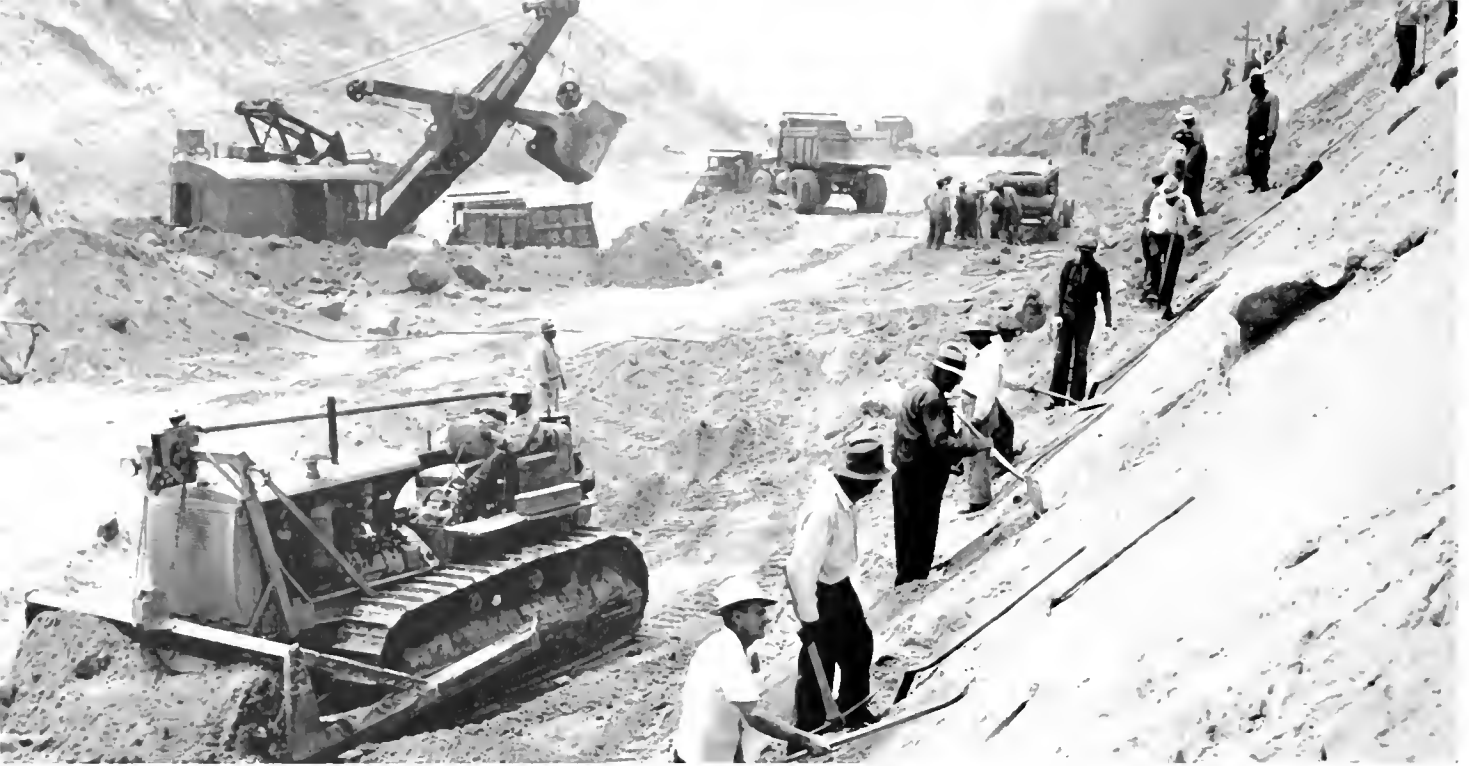
Big power shovels, tractors, bulldozers, trucks and some of 2,000 men engaged in building Arroyo Seco extension through Elysian Park
